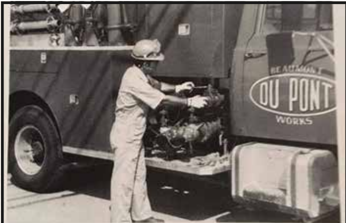
The plant's fire protection equipment is thoroughly inspected by Patrolman Ben Hughes, Jr.
